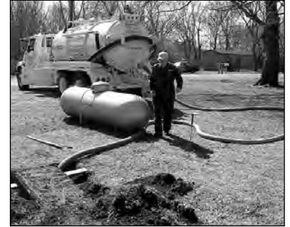
Legacy Septic Tank Program
